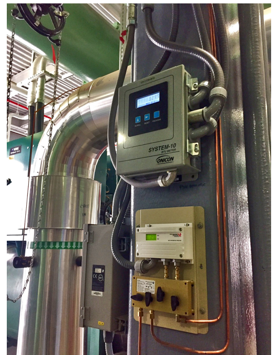
ONICON System-10 BTU Meter Installed in a Chiller Plant
