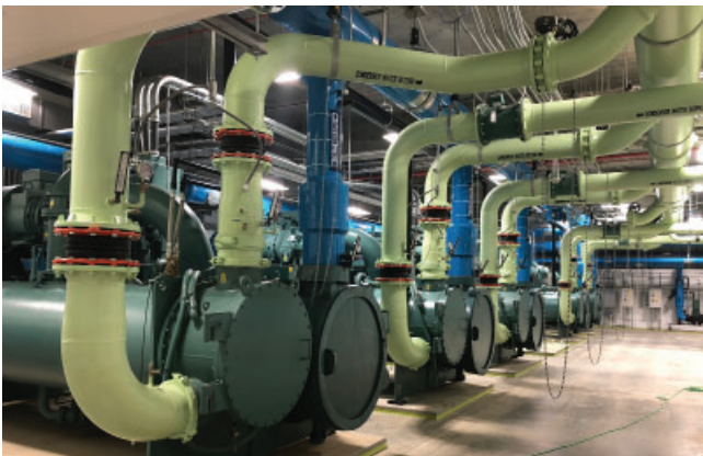
Supply and Return pipes inside a chiller plant
