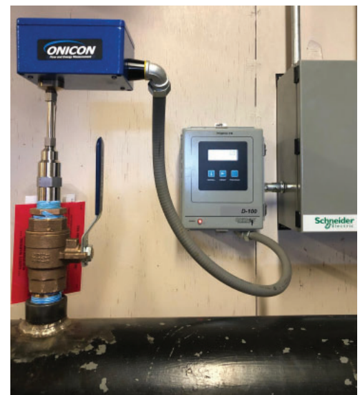
ONICON Flow and energy meters used to calculate energy usage.
